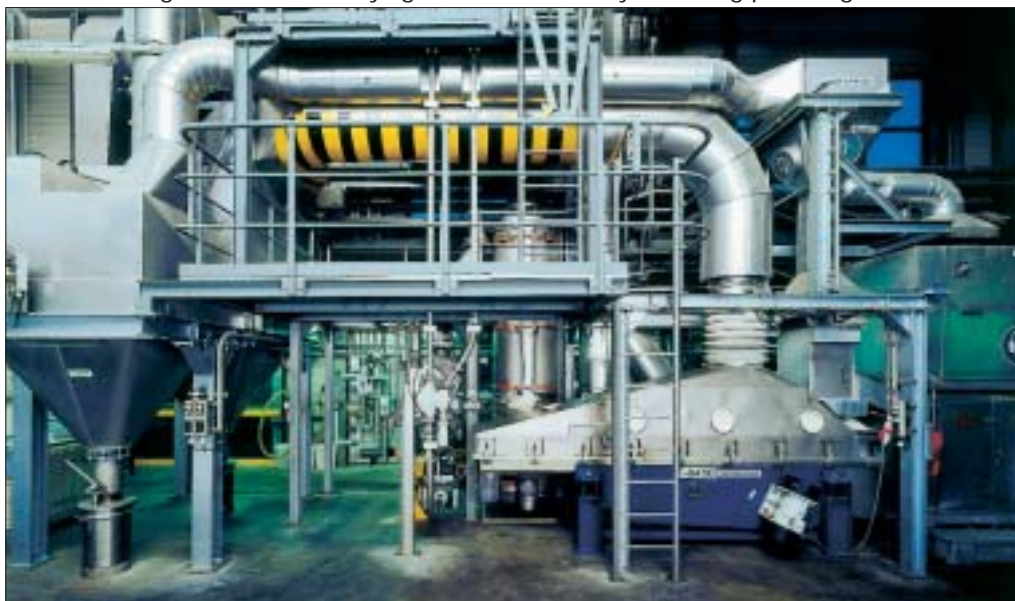
Figure 31 VSK 25-7/7 vibratory fluid-bed dryer with integrated screen and complete air-handling equipment, including a dust filter, for drying and simultaneously screening plastics granules
