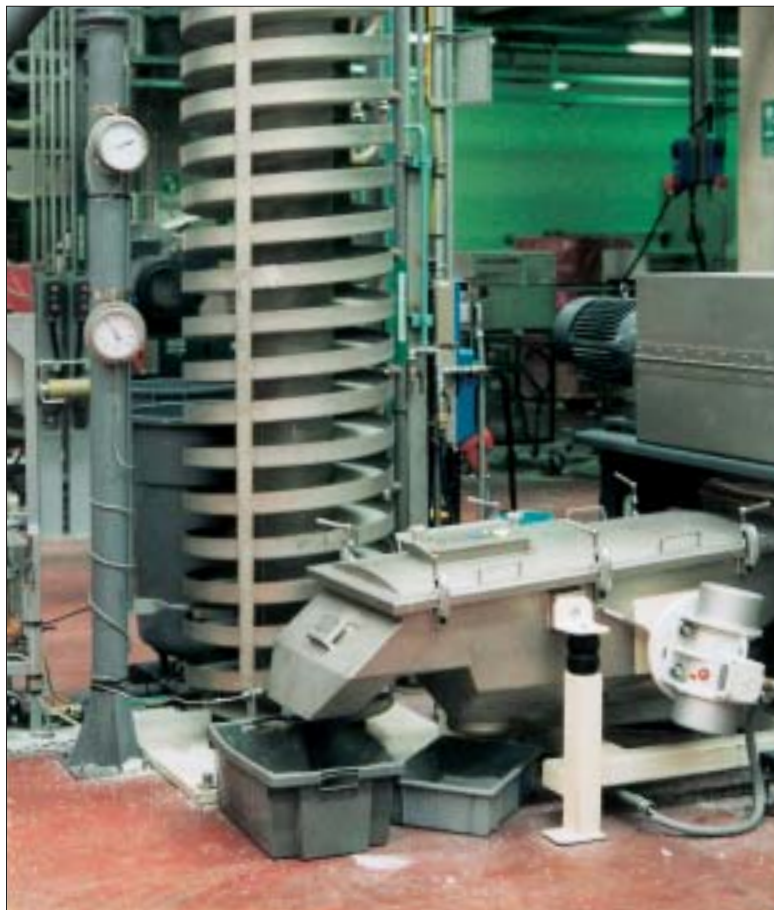
Figure 25 SRK screening machine in a granulating plant
